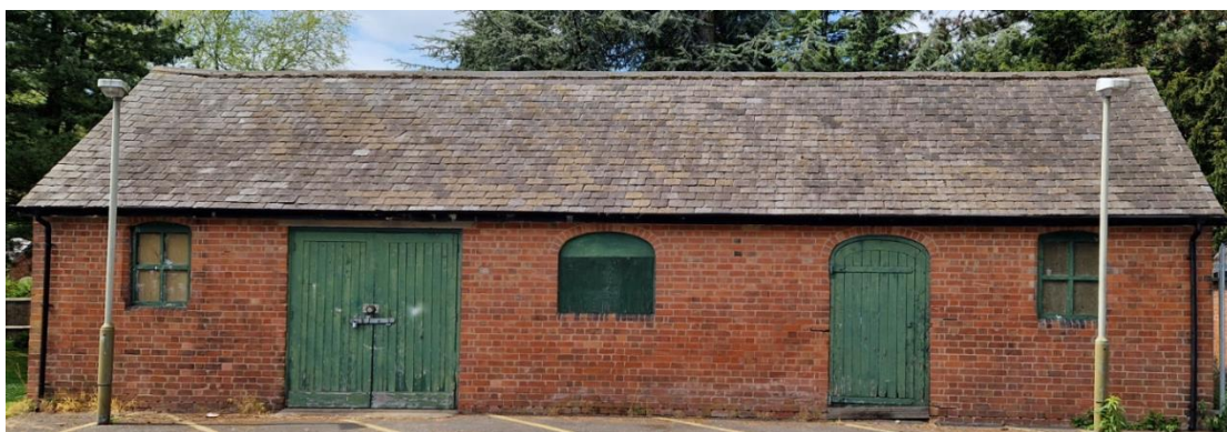
Former farm building in Evington Park with an attractive Welsh Slate Roof
